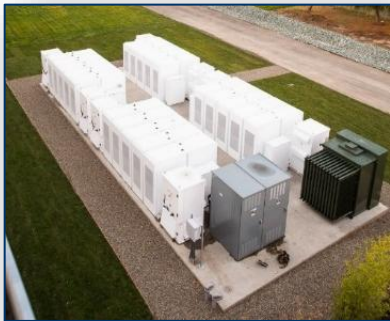
Battery Energy Storage Systems (BESS)
