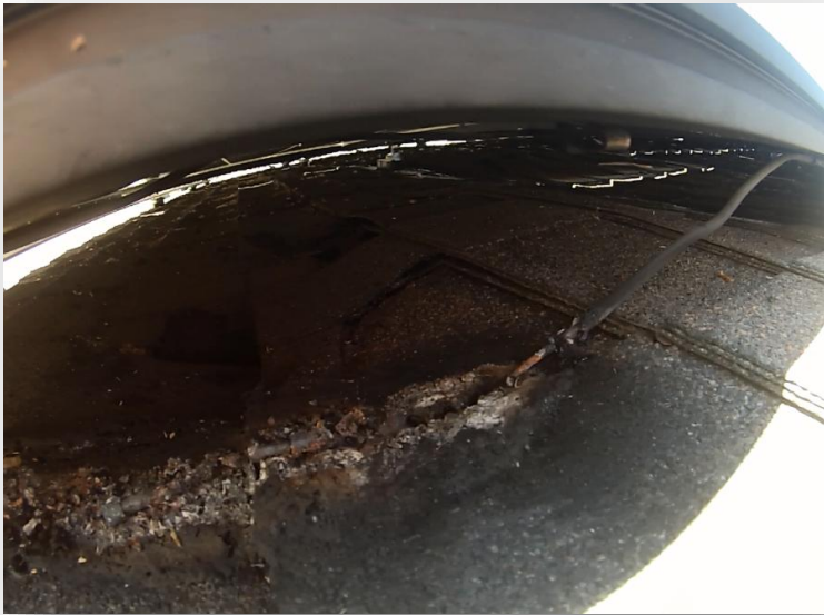
Fire caused by arc fault at loose connector
